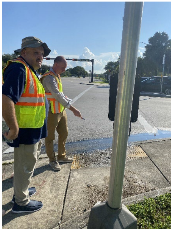
Poor curb condition at Hiatus Road intersection
