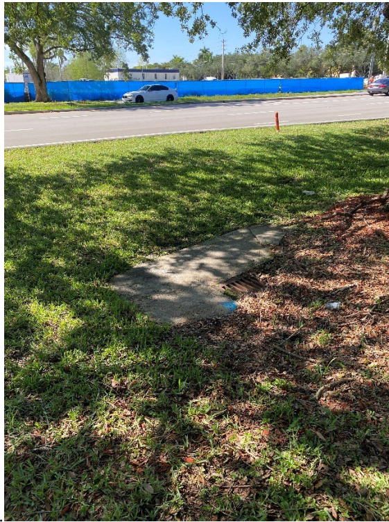
Clogged drainage inlet on eastern half of corridor
